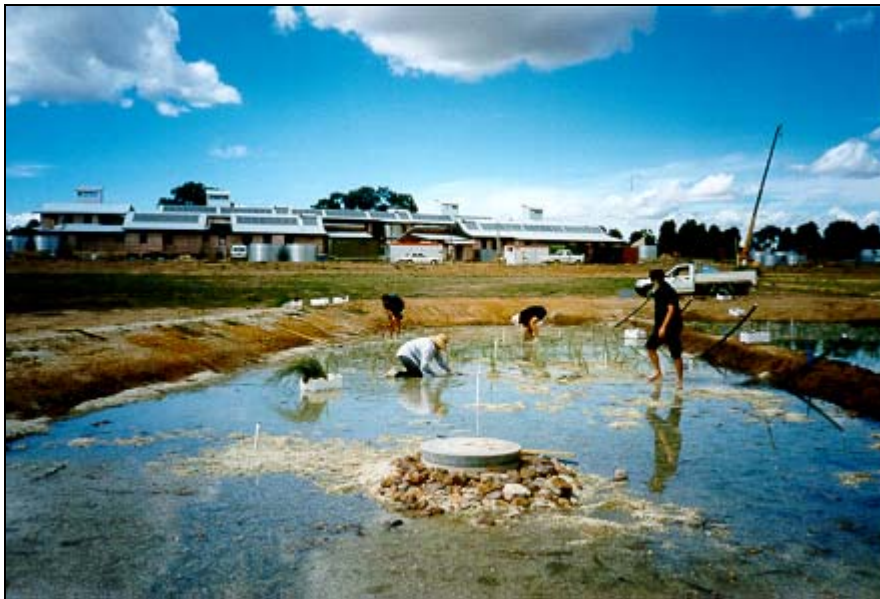
Establishment of SEIS Greywater Treatment Wetlands. The wetland is flooded above the gravel for initial planting to take place. Note the outlet sump in foreground.
