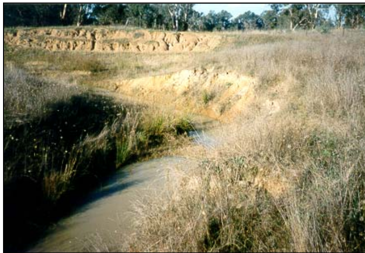
Erosion in Six-Mile Creek
